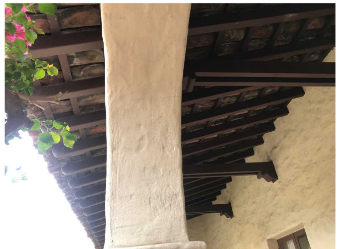
Exposed undersides of clay roof tiles on roof overhanging loggia. Wooden structural elements visible. Trusses appear to be decorative rather than functional.
